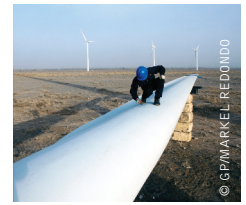
image A MAINTENANCE WORKER MARKS A BLADE OF A WINDMILL AT GUAZHOU WIND FARM NEAR YUMEN IN GANSU PROVINCE, CHINA.
