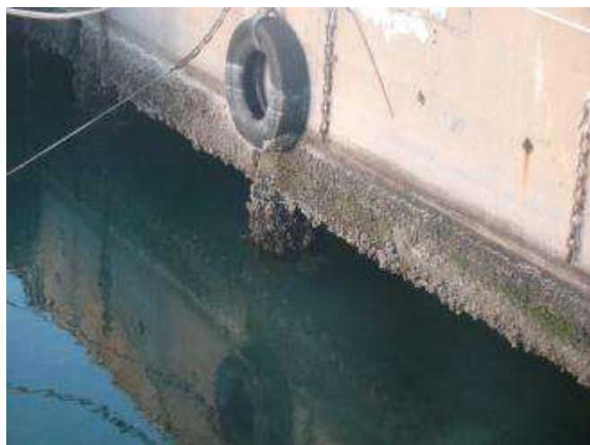
Figure 28: Lower section of quay showing sign of possible exfoliation of supports
