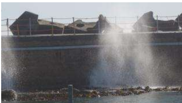
Figure 11: Blow through under main breakwater
