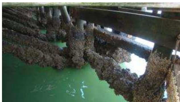
Figure 34: Underside of wooden jetty shows heavy encrustation and some rot
