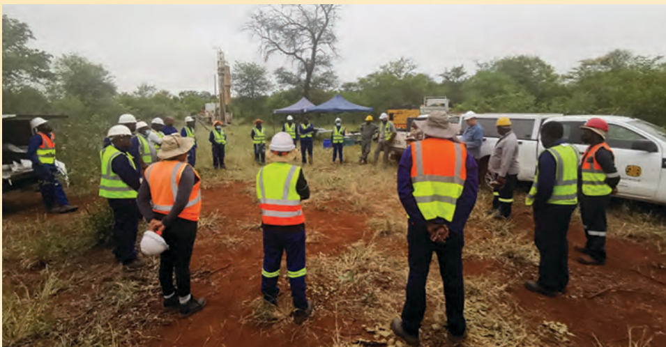
CGS team of scientists, drillers and technical assistants preparing themselves to start drilling a reverse circulation borehole in the Giyani Greenstone Belt.
