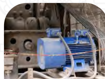
ELECTRIC MOTORS & DRIVES
